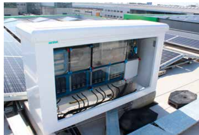
Dakopstelling verdelerkast Geyer.
